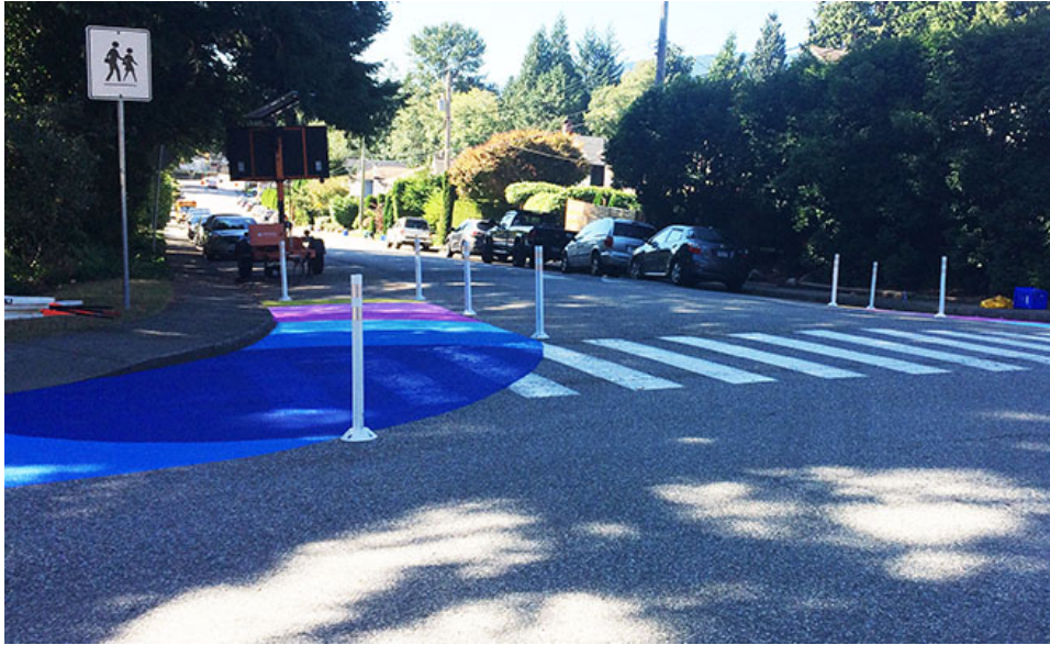
Corner bulges with flexible delineators and murals at Larson Ave and 28 th St
