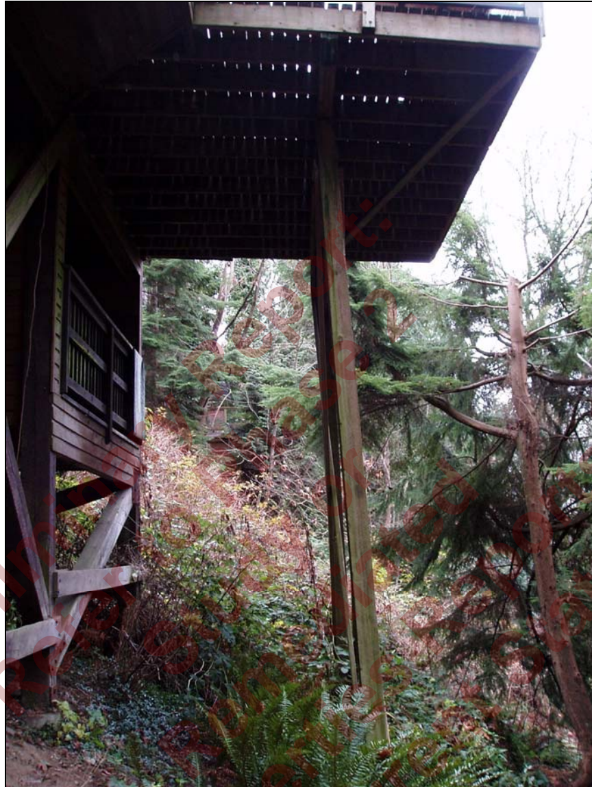
Plate 2: Note the displacement of the post supporting the deck on this structure (thought to be at 2101 Westview Drive). The crest of the ravine is located next to the base of these posts. The BC Hydro RoW is in the background of the picture.
