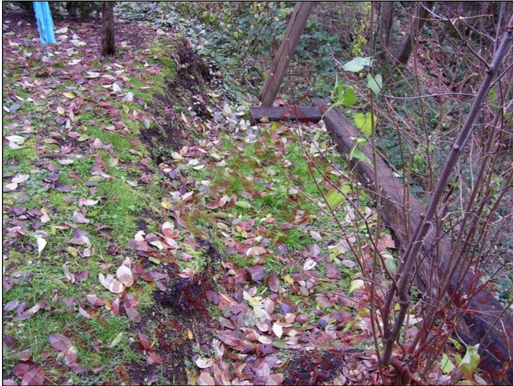
Plate 3: The separation behind the face of the retaining wall.
