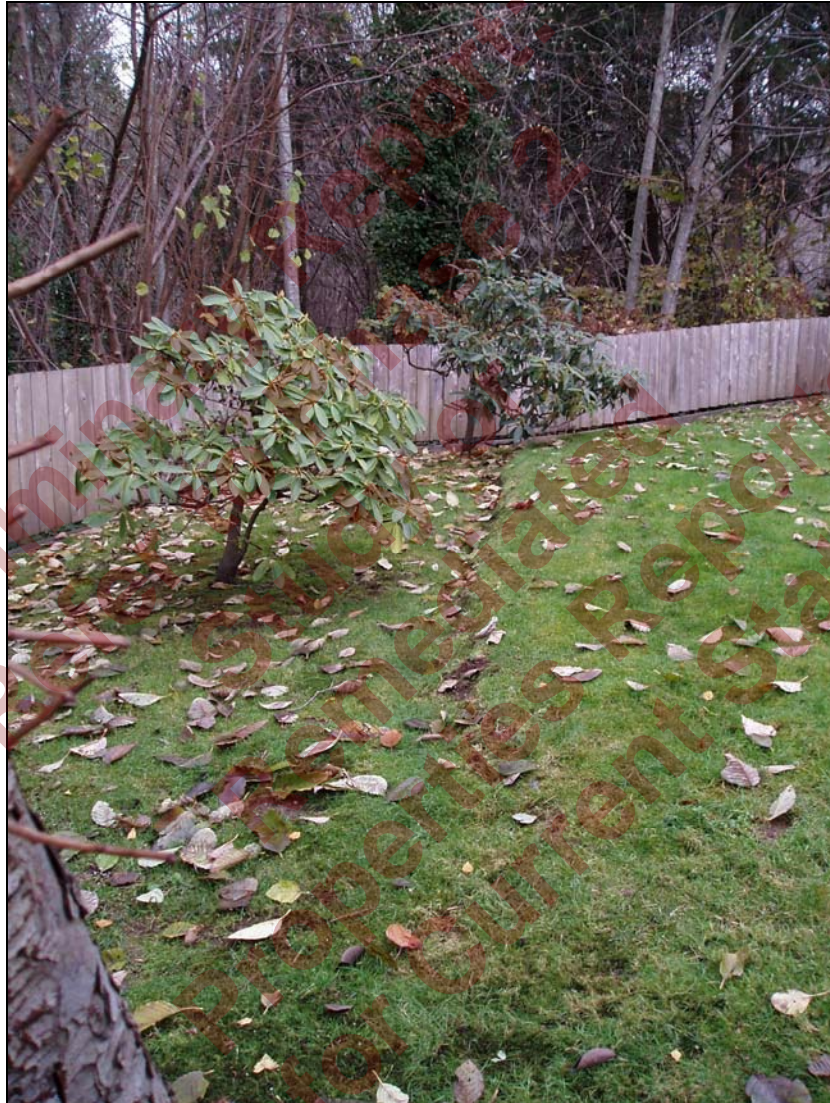
Plate 5: The tension crack and slumping fills at the rear of the lots from 1805 to 1821 Bewicke Ave. The crest of the ravine slopes is adjacent to the fence on the left side of the picture.
