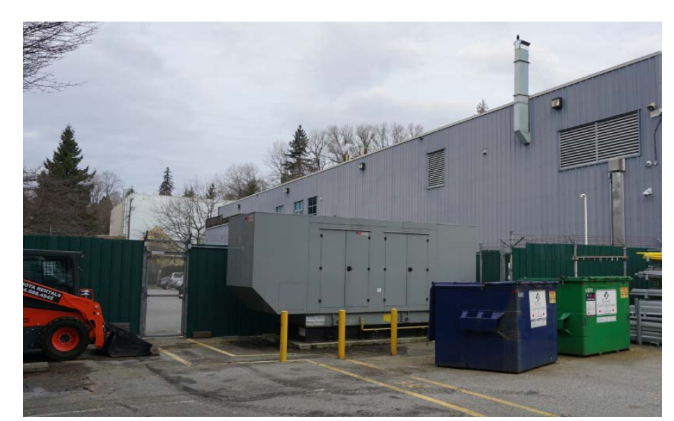
1 GENERATOR AND GATE / FENCE
