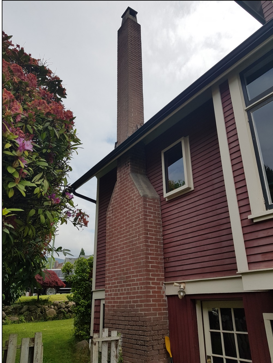
The end-wall chimney on the west elevation shows evidence of three different interventions at basement level.
