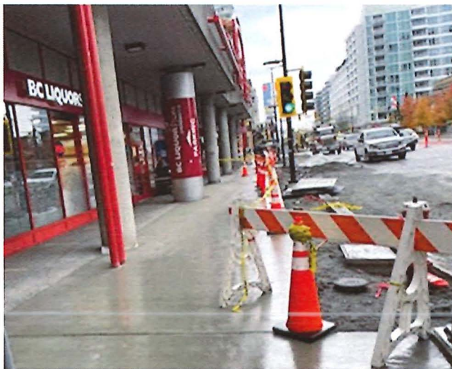
First sidewalk section on the 100 Block West is installed to support business operations.
